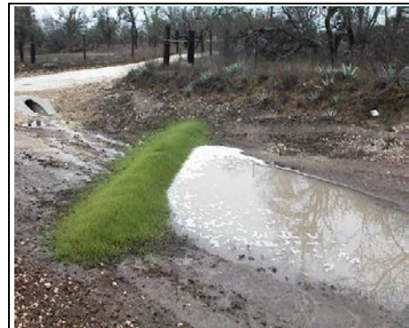
Vegetated compost filter berm. Note sediment on upstream side of berm and clear water on downstream side. Source: S. McCoy, Texas Commission on Environmental Quality.
